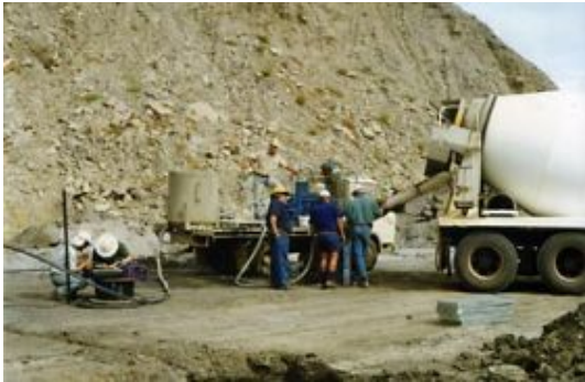
Preparing to cement an experimental geophone string in a borehole in Central Queensland. Image credit – CSIRO
