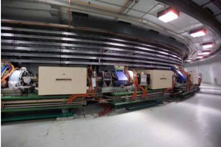
Equipment installation inside the Spallation Neutron Source ring tunnel. Image courtesy of Oak Ridge National Laboratory.
